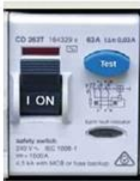
Household installed Safety Switch
